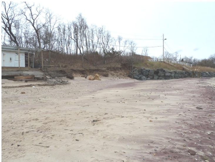
Figure 3. Soundview Avenue. An unprotected bluff blowout occurs at the east edge of a town-built revetment because the revetment is more resistant to erosion but is subject to being outflanked by erosion from the side. 12/26/2012 []
