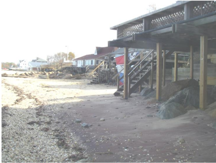
Figure 2. Soundview Avenue, Southold, west of town beach. Groins and bulkheads to the west inhibit the supply of sand with the result that the beach is lowered, allowing storm surges to attack residences. 11/12/2014
