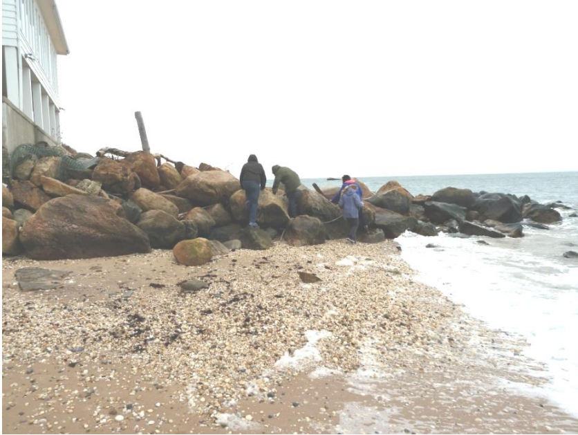
Figure 5. 21815 Soundview Avenue. Boulder groin blocks safe public passage along the beach, which is a violation of the public's right of lateral access. 12/26/2012
