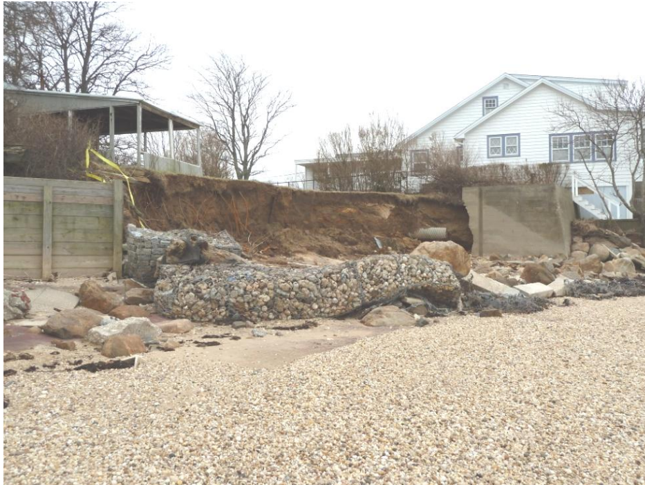
Figure 4. 21815 Soundview Avenue. Bluff blowout adjacent to a seawalled property that itself is threatened as erosion cuts back to outflank the seawalled property's foundation and also undermine a neighbor's unprotected residence. Notice the wired gabion placed to protect the bluff has been tossed aside by wave action. 11/12/2014
